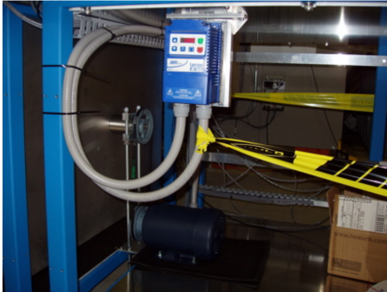
Figure 2-1. Photograph of the VFD (blue device) and blower motor (below). Power supplies to the VFD are through conduits supplied by the electrical contractor.
