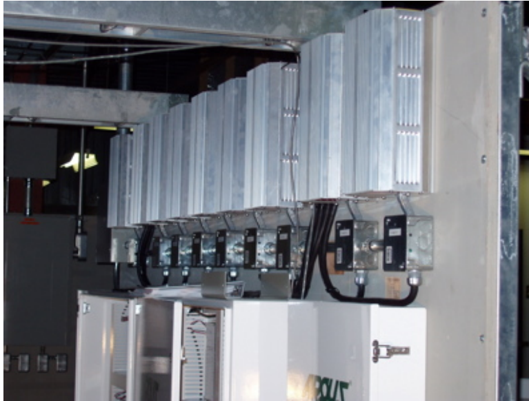
Figure 2-3. Photograph of the lighting system ballasts, contactors (below) and Argus I/O panels. The mounting frame for the ballasts as installed at the CESRF is also shown.
