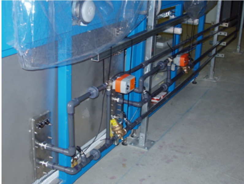
Figure 4-1 Photograph of the water supply service lines to the coils. The hot water coil (left) and chilled water coil (right) are connected to the proportional valve (orange device) and pressure regulator (brass device). Connection to and from facility supply is made to the pressure regulator and from the proportional valve, respectively.
