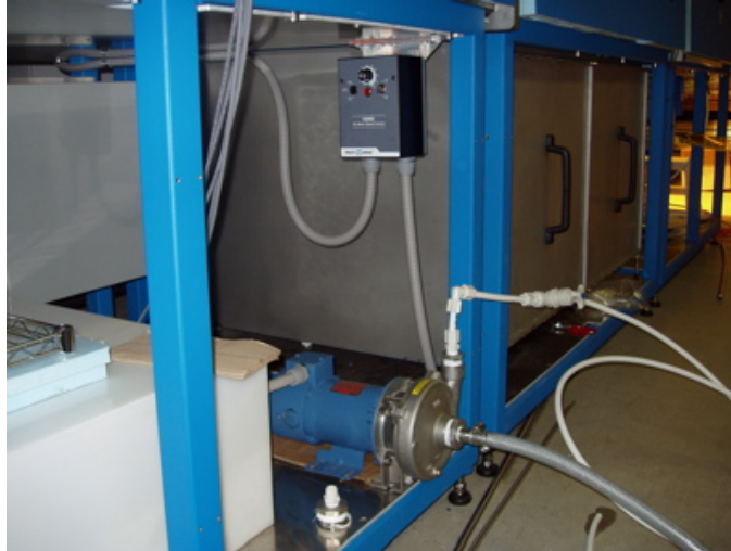
Figure 2-2. Photograph of the irrigation pump and manual speed controller (above). Power supplies to the pump are through conduits supplied by the electrical contractor.
