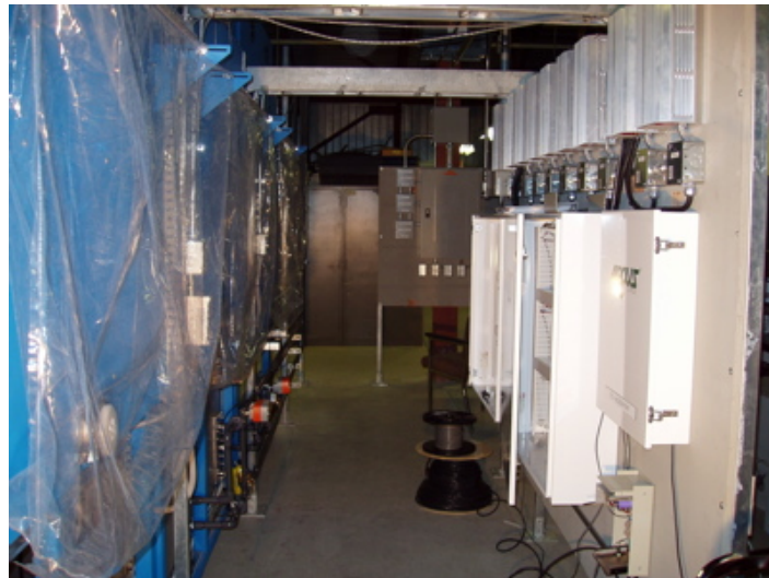
Figure 3-2. Photograph of mounting frames for ballasts in relation to the chamber. Shown are also the passive pressure compensation bladders.
