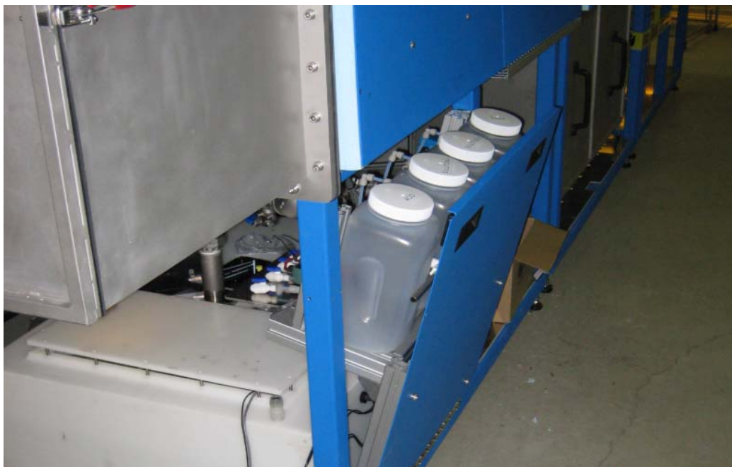
Illustration 8: Location of the stock solution reservoirs. Note that the front panel tilts forward to allow access.
