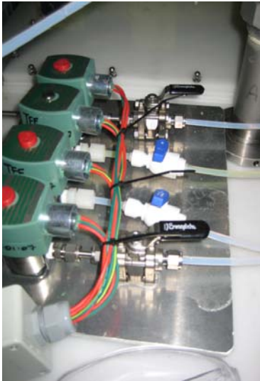
Illustration 11: Stock solution isolation valves are located on top of the NDS main reservoir.
